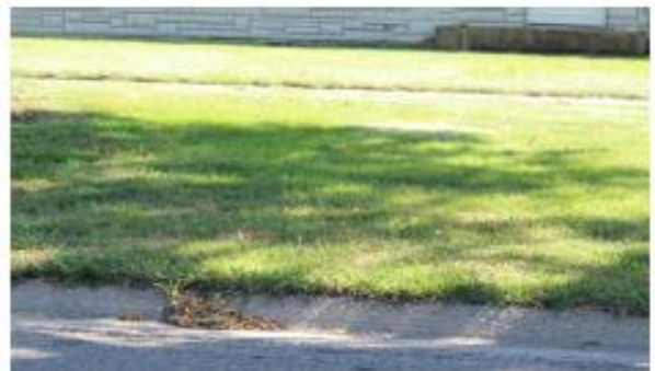
Photo 5: Vegetation gathering due to poor drainage in gutter
