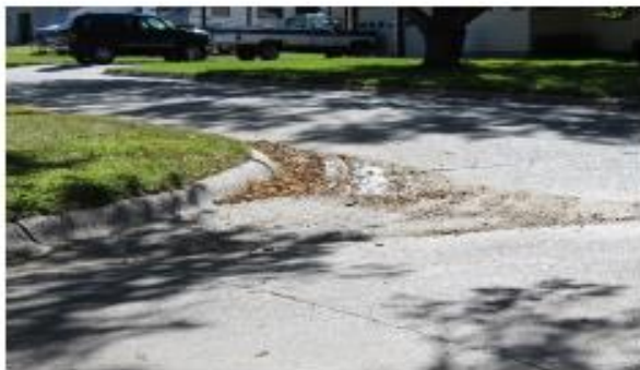
Photo 2: Poor drainage in gutter
