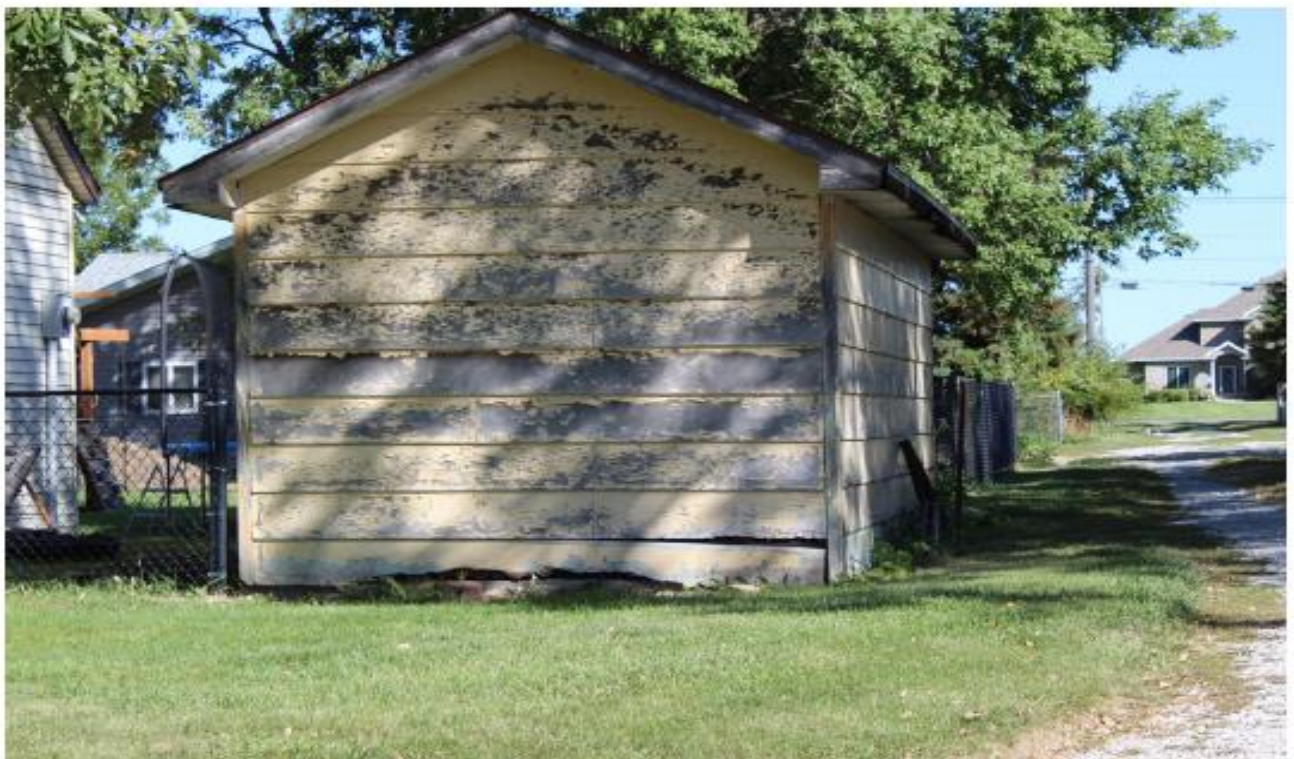
Photo 1: Structure in Poor Condition
